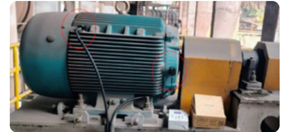
Figure 1: MOVUS Sensors on hot combustion blower
