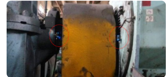
Figure 2: MOVUS Sensors on coke oven pump
